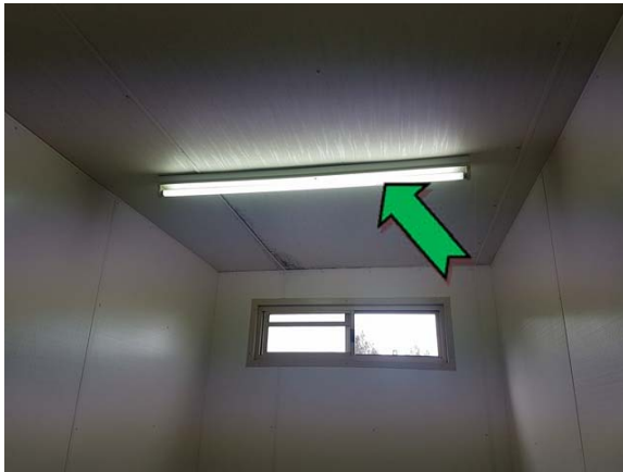
Photo 3. Interior, throughout, double tube fluorescent light fitting – suspected non PCB-containing capacitors.
