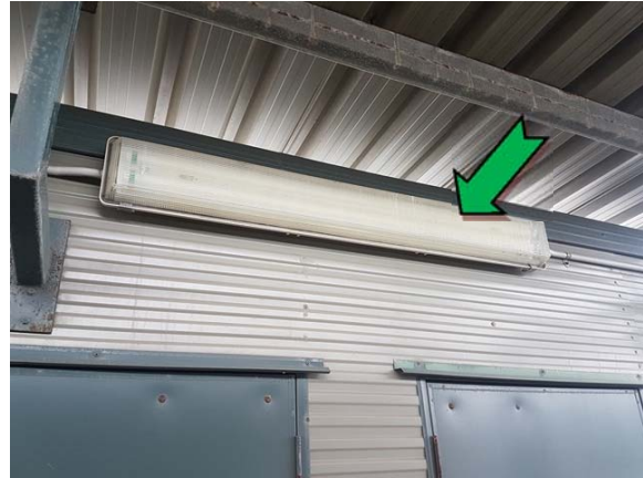
Photo 2. Exterior, throughout, double tube fluorescent light fitting – suspected non PCB-containing capacitors.
