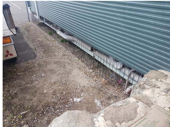
Photo 4. No access to the subfloor at the time of the Assessment.
